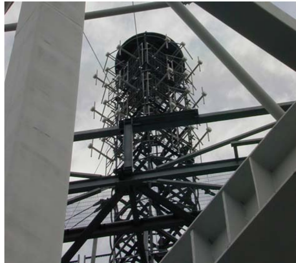
Figure 3. Original FM master antenna from Shively Laboratories.
