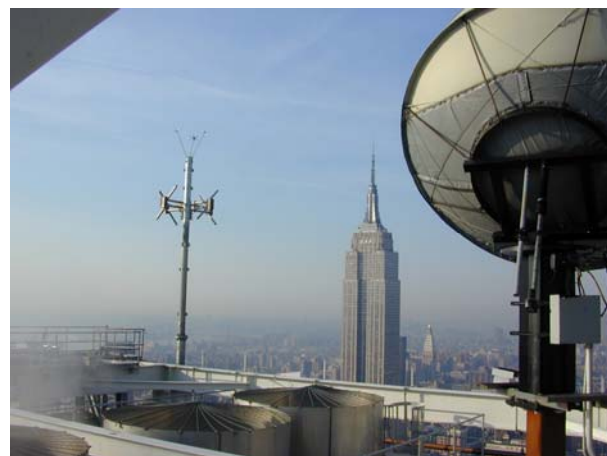
Figure 4. The FM backup antenna mounted near the southeast corner of the 4TS building. The Empire State Building is seen in the distance.
