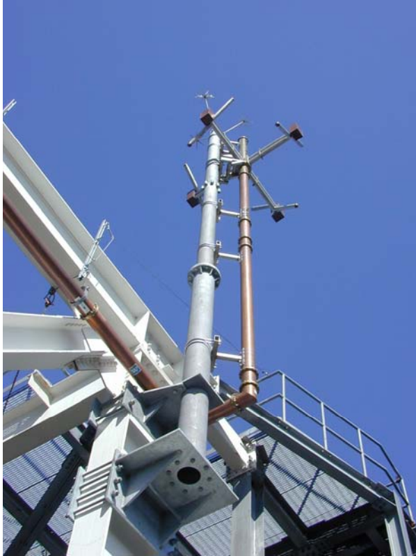
Figure 5. Closeup photograph of the Lindenblad FM backup antenna at the 4TS facility mounted to the steelwork of the eastern facing 4TS sign.
