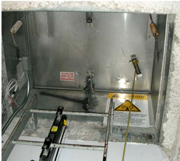
Figure 11. RF Tower Caution sign installed on tower access hatch.
